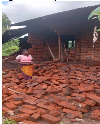
Regina's collapsed house
